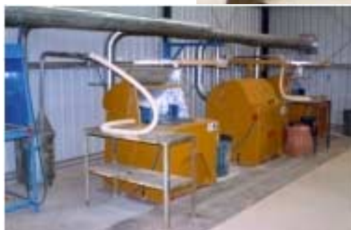
LM5 mills installed at a commercial assay laboratory in Kalgoorlie, Western Australia. Note this customer's preference to install their own (white coloured) flexible vacuum hoses for final bowl cleaning and their introduction of a coarse dust trap between the mills and their dust extraction ducting
